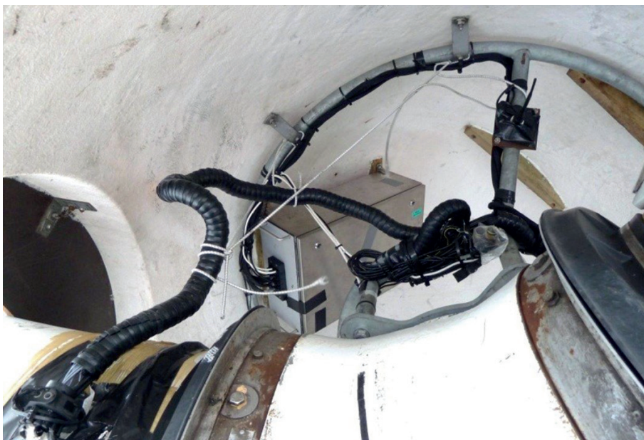
The data acquisition hardware was mounted in a single rack and secured in a waterproof box in the rotor housing. A slip ring was used for power transmission. Data was transmitted wirelessly to the PC in the tower, and synchronized using an IrigB time code
